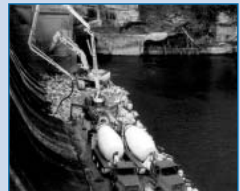
Cooperation and organization of efforts allowed for the successful emergency stabilization of the Rapidan Dam.
